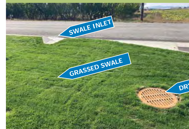
Shallow dry wells should be installed away from curb cuts in order to pre-treat the water before infiltrating into the well.
